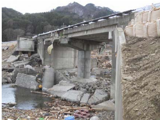
Photo-19 Washed-away main girders (H-shape steel girders) of bridge-side pedestrian bridge (Rte. 45, pedestrian bridge at Namiita Bridge (inbound side), Otsuchi Town, Iwate Pref.)
