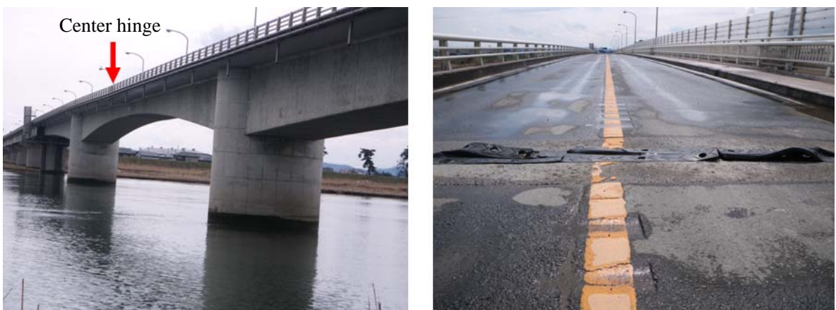
Photo-3 Displacement at the center hinge of rigid-frame bridge (principal local road, Shiogama-Watari Line; Yuriage Bridge, Natori City, Miyagi Pref.)
