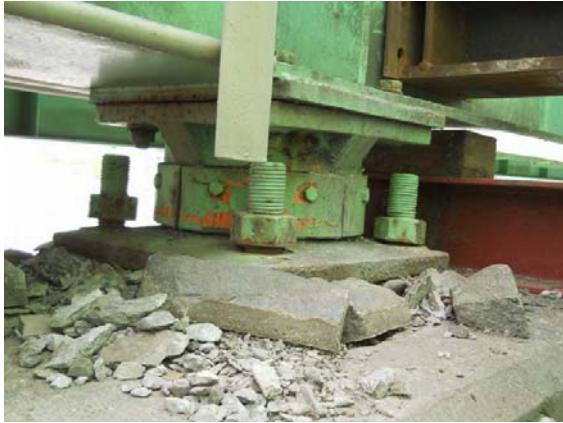
Photo-9 Cracking/loss of shoe seat mortar (Rte. 45, pedestrian bridge at Tenuoh Bridge, Ishinomaki City, Miyagi Pref.)
