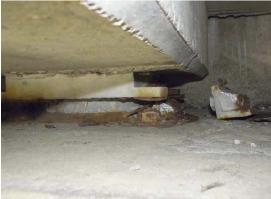
Photo-26 Deformation/fracture of bearing side block (Rte. 45, Utatsu Bridge, Minamisanriku Town, Miyagi Pref.)
