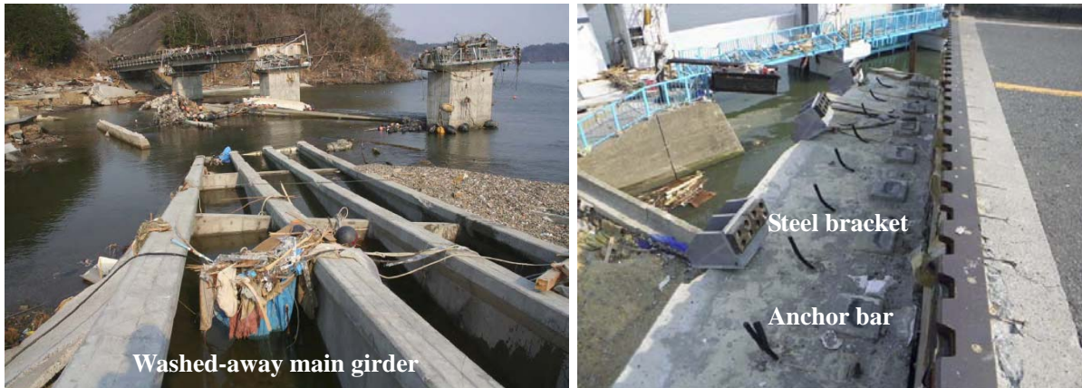
Photo-15 Washed-away main girders (PCT girders) (Rte. 45, Utatsu Bridge, Minamisanriku Town, Miyagi Pref.)
