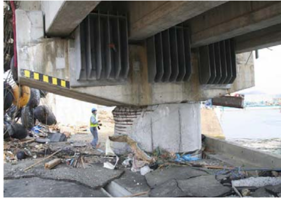
Photo-22 Damaged pier (Rte. 45, Utatsu Bridge, Minamisanriku Town, Miyagi Pref.)
