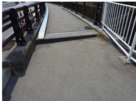
Difference of surface level in pedestrian section (difference of more than 2 cm)
