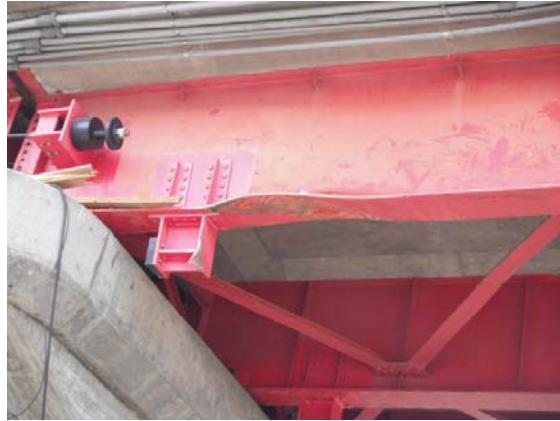
Photo-20 Main girder deformed by impact of floating debris (Rte. 45, Katagishi Bridge, Kamaishi City, Iwate Pref.)
