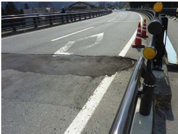
Difference of surface level in roadway section (after emergency repair by construction of ramp)
