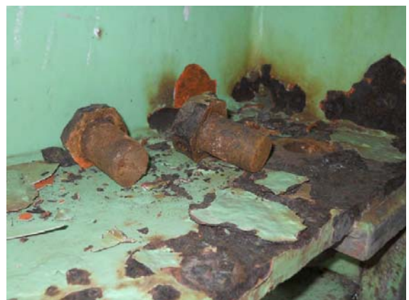
Photo-8 Fracture of set bolts (Rte. 45, Tennoh Bridge, Ishinomaki City, Miyagi Pref.)
