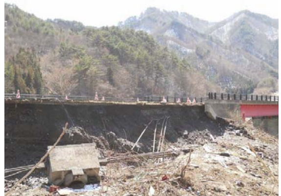
Photo-29 Scouring of approach embankment (Rte. 45, Toyasaka Bridge, Kamaishi City, Iwate Pref.)
