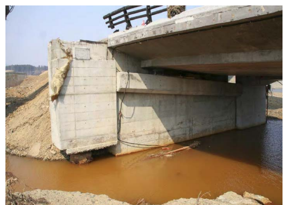
Abutment of pedestrian bridge showing an exposed foundation pile
