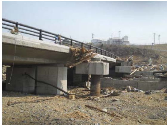
Photo-18 Washed-away main girders (PCT girders) of bridge-side pedestrian bridge (Rte. 45, pedestrian bridge at Sodeogawa Bridge (outbound side), Kesenuma City, Miyagi Pref.)
