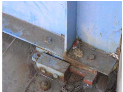
Abnormal gap (movable bearing)
