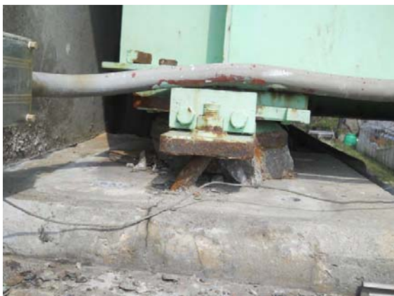
Photo-7 Deformation of anchor bolts (Rte. 45, pedestrian bridge at Tennoh Bridge, Ishinomaki City, Miyagi Pref.)
