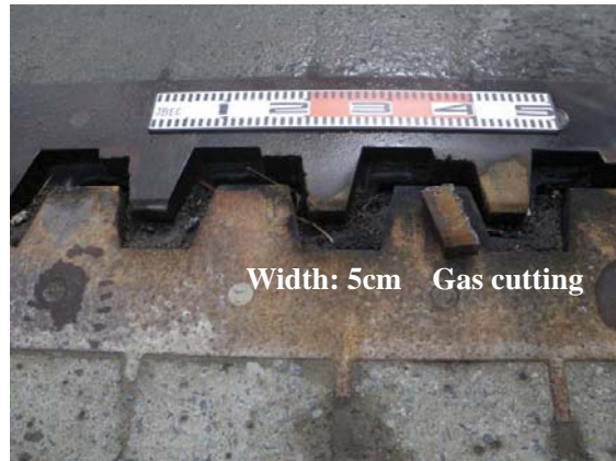
Photo-13 Abnormal expansion gap of expansion joint perpendicular to bridge axial direction (principal local road, Shiogama-watari Line; Yuriage Bridge, Natori, Miyagi Pref.)
