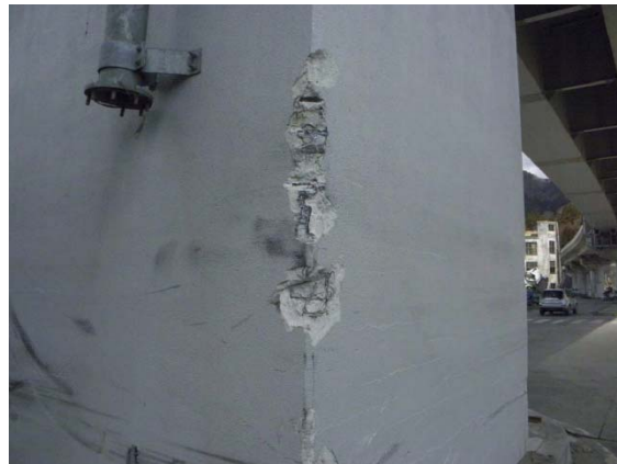
Photo-23 Damage to pier by impact of floating debris (Rte. 45, Kamaishi Viaduct, Kamaishi City, Iwate Pref.)
