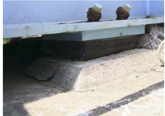
Photo-27 Deformation/pulling out of anchor bolts (Rte. 45, pedestrian bridge at Osawa No.2 Bridge (inbound side), Kesenuma City, Miyagi Pref.)
