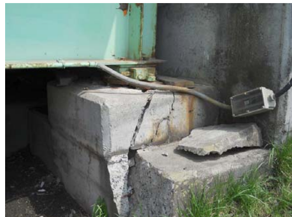
Photo-5 Cracks in abutment (Rte. 45, pedestrian bridge at Tennoh Bridge, Ishinomaki City, Miyagi Pref.)
