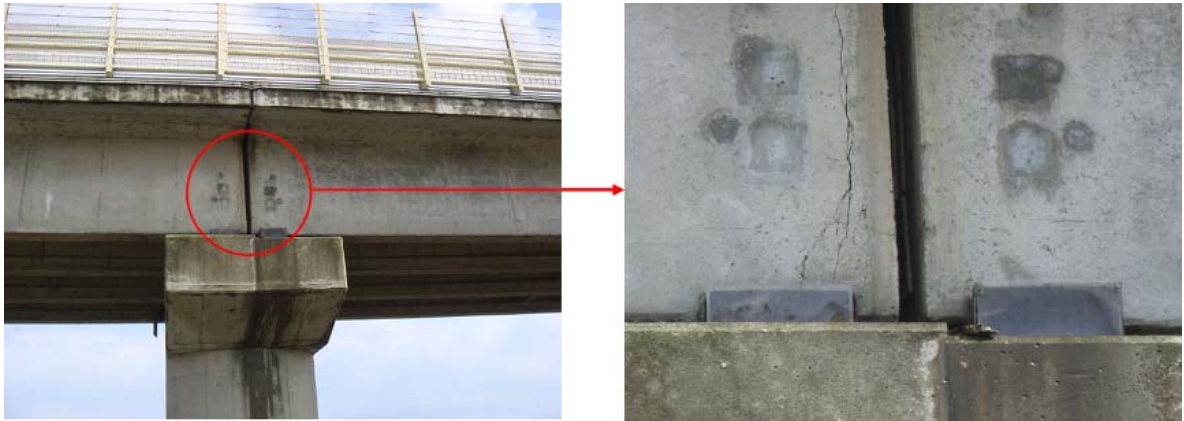
Photo-1 Cracking of ends of main girders (supporting point) (principal local road, Shiogama-Watari Line; Yuriage Bridge, Natori City, Miyagi Pref.)
