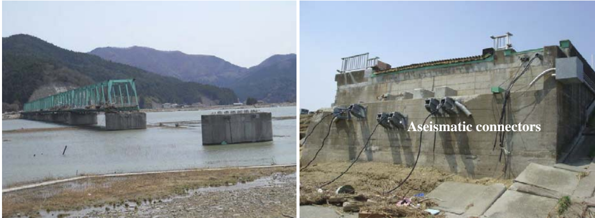
Photo-17 Washed-away main trusses (Rte. 398, Shin-Kitakami Bridge, Ishinomaki City, Miyagi Pref.)
